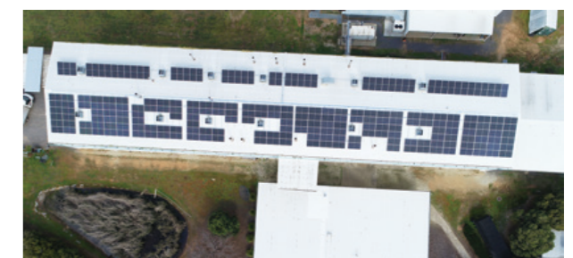
Solar panels installed at ITO EN AUSTRALIA PTY. LIMITED
